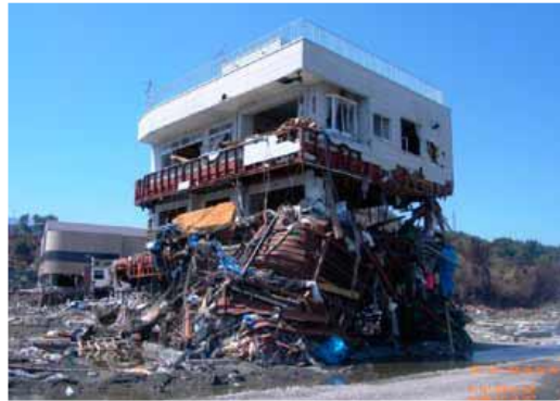
Figure 4. Floating debris trapped 3 storey building structure.
